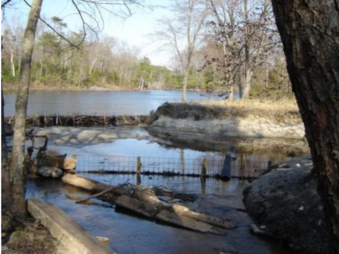
Figure 14. A diversion dam (left center), a Round Fence™ (lower right), a Castor Master™ (lower right) and receiver fence (lower center) installed in November 2005 to protect three culverts directing water underneath Route 616 on Newton's Pond in Westmoreland County, Virginia.
