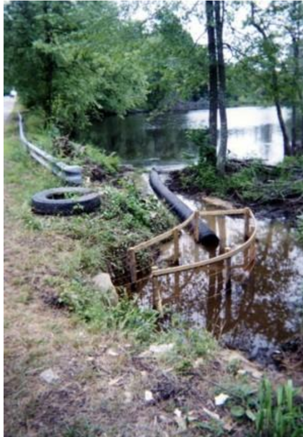
Figure 21. A Beaver Deceiver™ installed in June 2004 to protect a culvert directing water underneath Route 630 on Second Swamp in Prince George County, Virginia. A Castor Master™ (center) and a Round Fence™ (beneath the surface of the water and attached to the upstream end of the Castor Master™) were attached to the upstream end of the Beaver Deceiver™ to augment water flow if beavers attempted to dam the fence.
