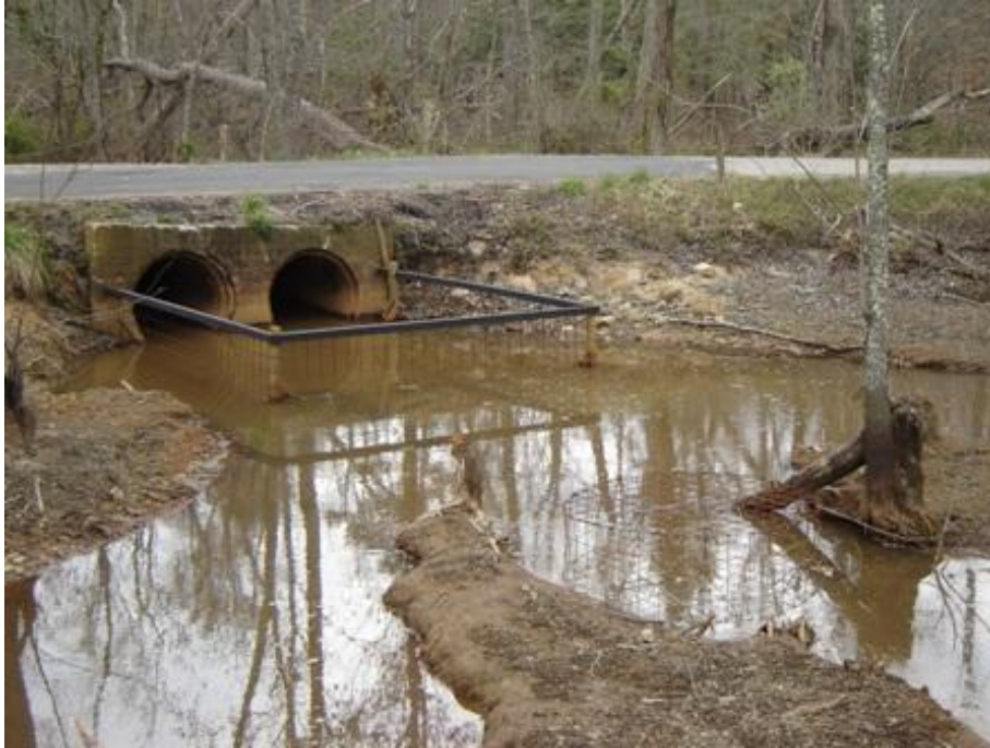
Figure 11. A Beaver Deceiver™ installed in November 2005 to protect two culverts directing water underneath Route 606 on Briary Swamp in Middlesex County, Virginia. A Round Fence™ (bottom center) and a Castor Master™ (beneath the surface of the water between the Round Fence™ and the Beaver Deceiver™) were attached to the upstream end of the Beaver Deceiver™ to augment water flow if beavers attempted to dam the fence.
