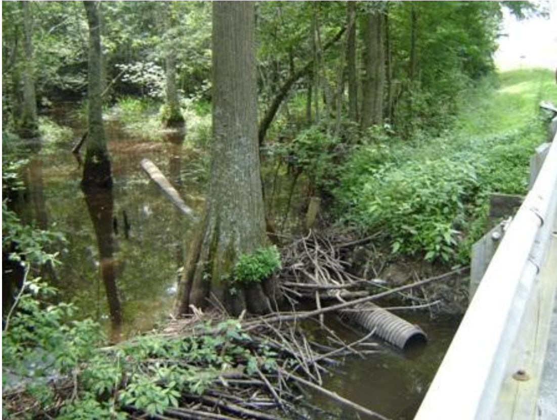
Figure 8. A Round Fence™ (top left) and a Castor Master™ (located beneath the surface of the water between the Round Fence™ and the existing beaver dam) were installed in June 2004 to protect a bridge directing water underneath Route 612 on Corrowaugh Swamp in Isle of Wight County, Virginia.
