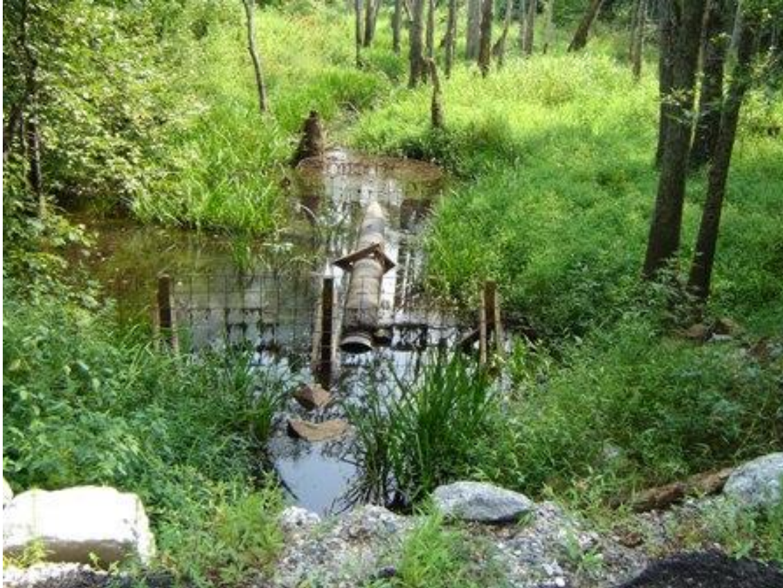
Figure 17. A Round Fence™ (top center) and a Castor Master™ (between the Round Fence™ and the receiver fence) attached to the upstream side of a receiver fence installed in May 2005 to protect a culvert directing water underneath Route 630 on Swift Creek in Chesterfield County, Virginia.
