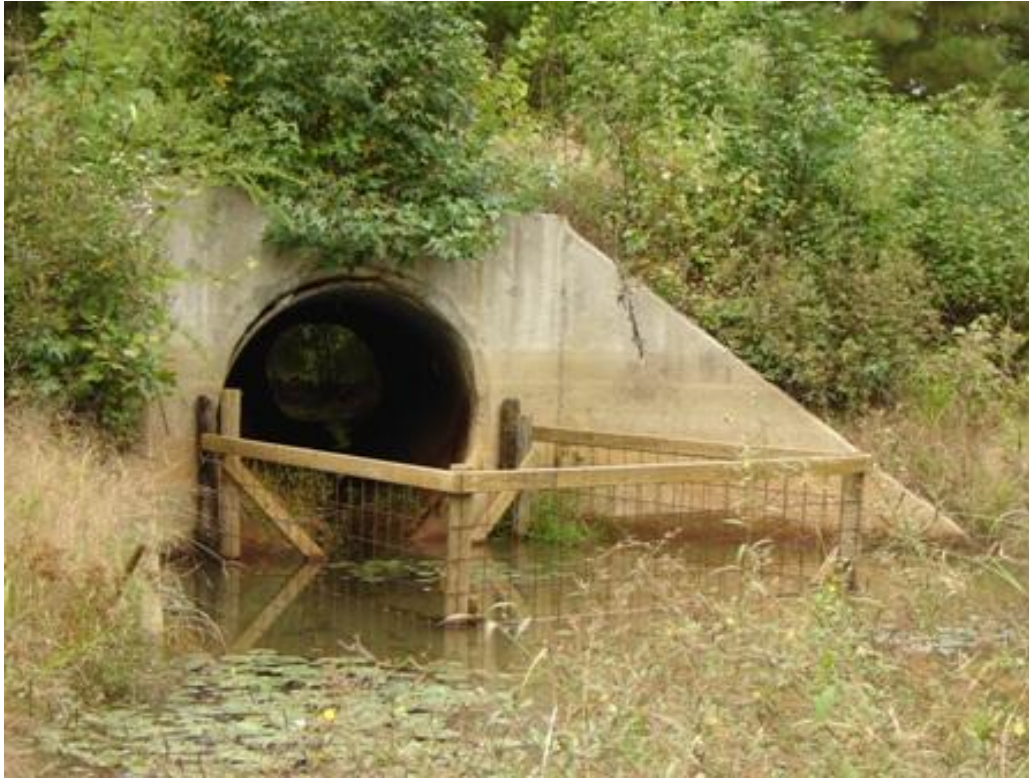
Figure 20. A Beaver Deceiver™ installed in May 2005 to protect culvert directing water underneath Route 1102 on Blackwater Swamp in Prince George County, Virginia.
