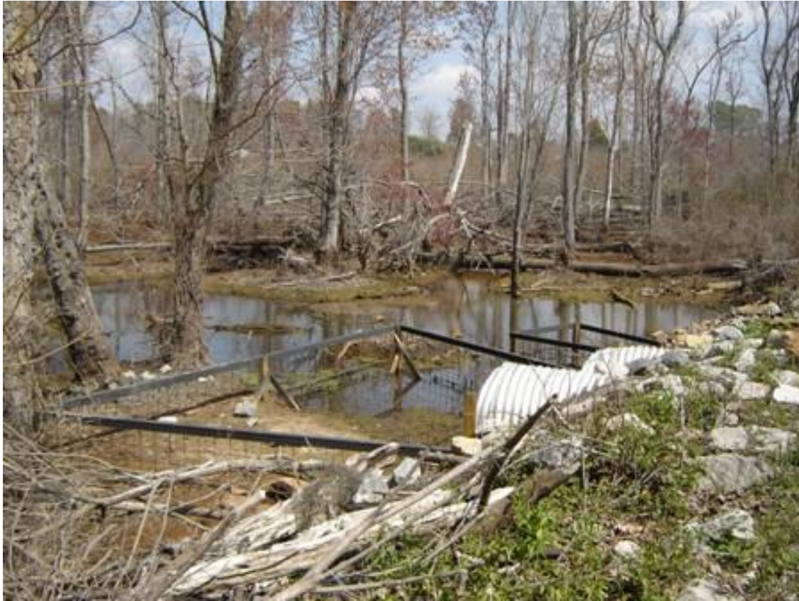
Figure 10. Two Beaver Deceivers™ installed in November 2005 to protect two culverts directing water underneath Route 619 on Craney Creek in Gloucester County, Virginia.
