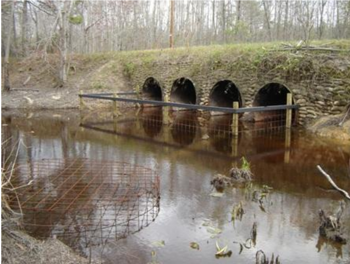
Figure 13. A Beaver Deceiver™ installed in November 2005 to protect four culverts directing water underneath Route 639 on Pope's Creek in Westmoreland County, Virginia. A Round Fence™ (bottom left) and a Castor Master™ (beneath the surface of the water between the Round Fence™ and the Beaver Deceiver™) were attached to the upstream end of the Beaver Deceiver™ to augment water flow if beavers attempted to dam the fence.
