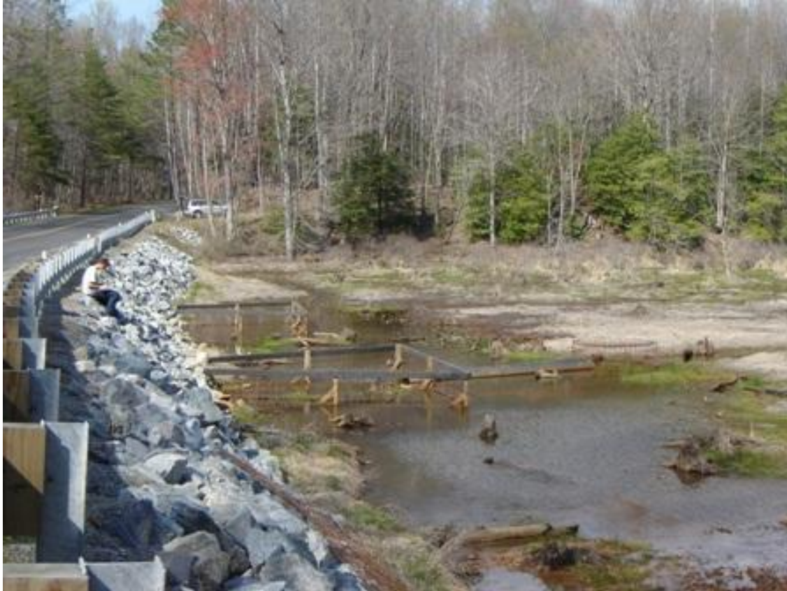
Figure 12. Two Beaver Deceivers™ installed in January 2005 to protect two culverts directing water underneath Route 624 on Pope's Creek in Westmoreland County, Virginia. A Round Fence™ (right center) and a Castor Master™ (between the Round Fence™ and the large Beaver Deceiver™) were attached to the upstream end of one Beaver Deceiver™ to augment water flow if beavers attempted to dam the fences.
